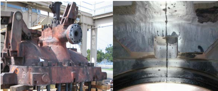
Steam Turbines cracks, steam cuts.....
